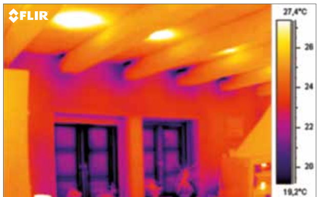
The thermal image shows thermal bridges between the roof beams and adjacent walls.
