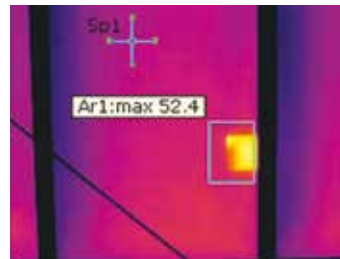
This thermal image shows a hot spot due to cell breakage in a standard 60 cell module.
